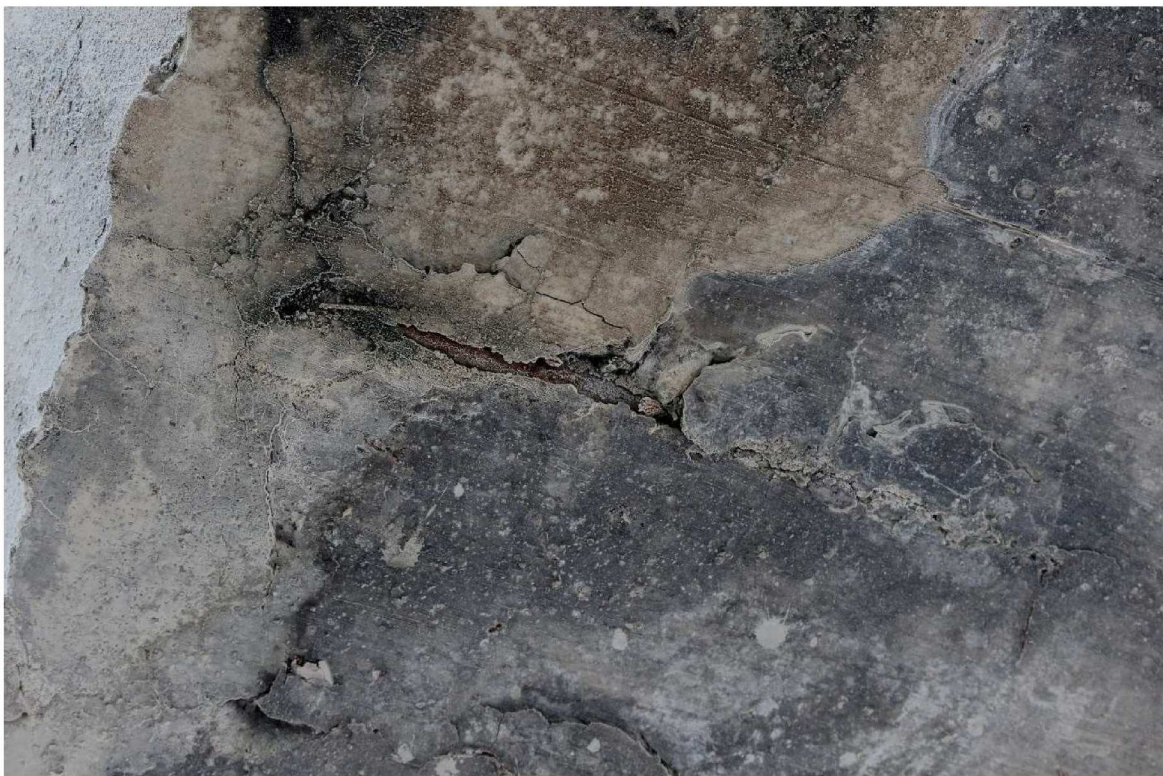
Figure 3.2. Poor concrete structure condition
