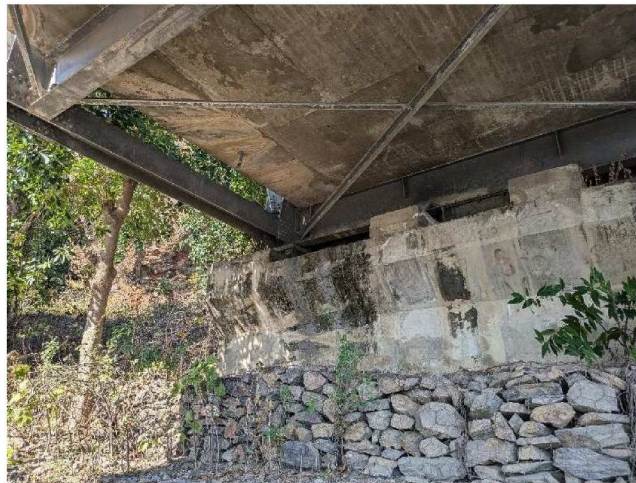
Figure 2.1. Initial damage and repair application to the concrete structure.
