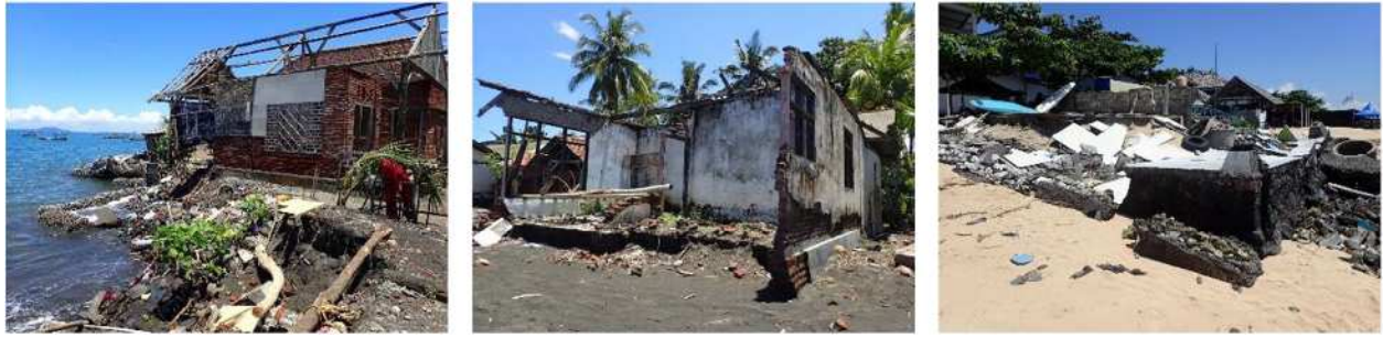
Figure 3-11. Destroyed coastal infrastructure in Bali Province due to erosion in sandy shores in Jembrana and Badung Regencies. (Source: field survey, 10—19 March 2023).
