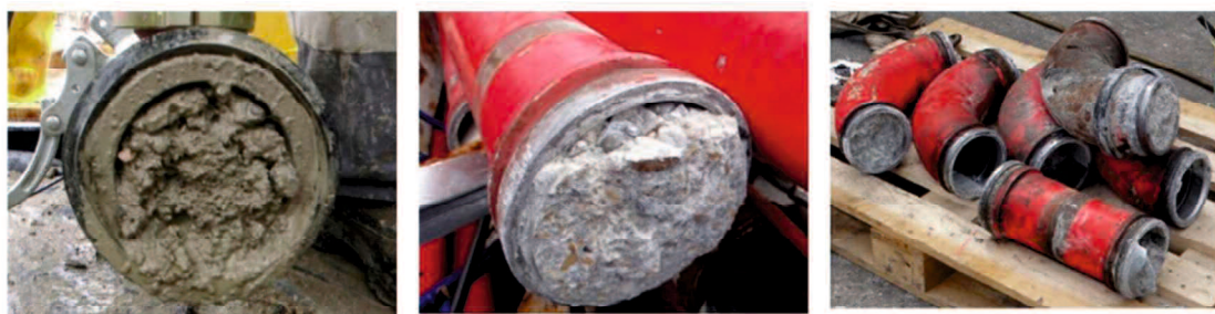
Fig. 1.2 Concrete blockage in pipeline
