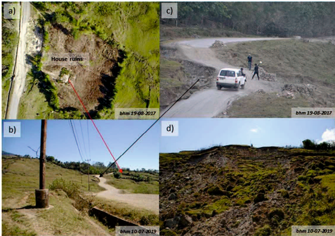
Figure 2.6. Evidence of ground deformation and its impact: a) house ruins, b) electrical pole that moved and tilted, c) degraded road conditions, and d) small landslide induced by an earthquake
