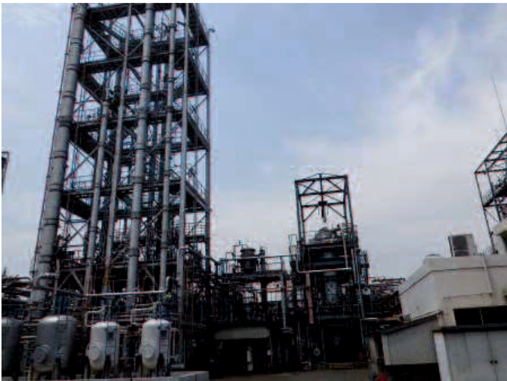
Fig. 5-2 Whole view of CPME plant
