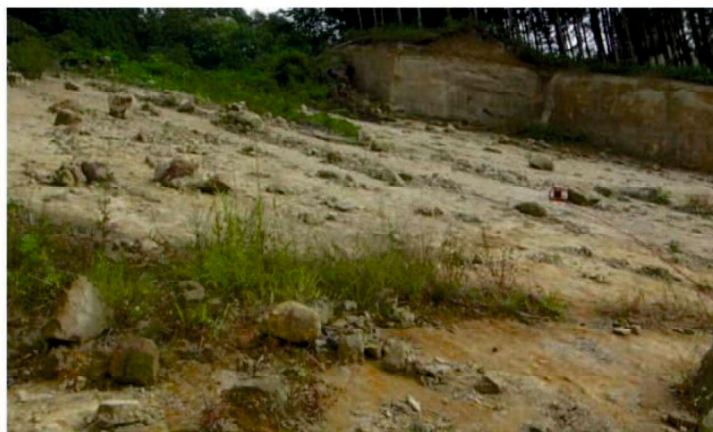
Figure 2.8 Sliding surface in sandstone in Niigata Prefecture (Suzuki et al., 2012)
