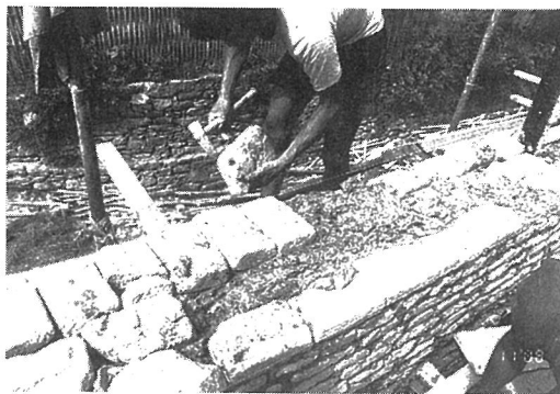
Photo. 3.6 Construction of a mud-stone house in Dharan Bazaar; cementing stones with mud-mortar
