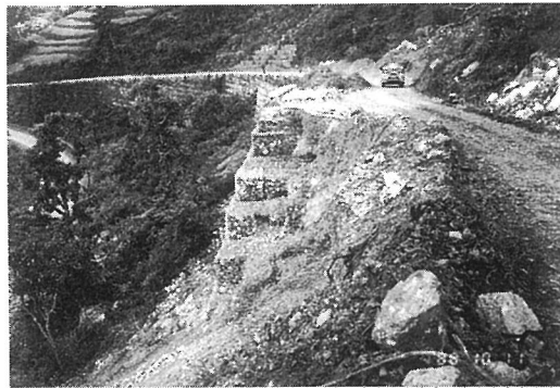
Photo. 3.70 Road damaged by a landslide
