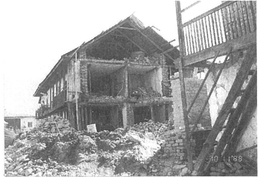
Photo. 3.37 Damage to the gable wall of a brick masonry building; example 2, Dhankuta Bazaar, Nepal
