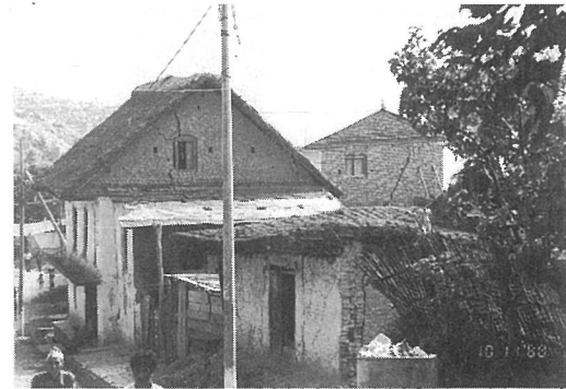
Photo. 3.39 Damage to the gable wall of a brick masonry building; example 4, Dhankuta Bazaar, Nepal
