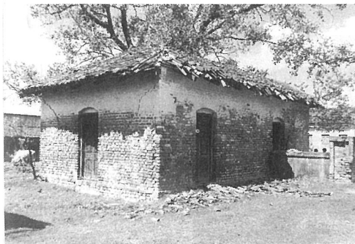
Photo. 3.14 A damaged kiosk in the backyard of the Darbhanga District Headquarters Office, Darbhanga, India
