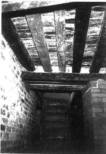
Photo. 3.3 Interior view of the floor slab system of a brick masonry building
