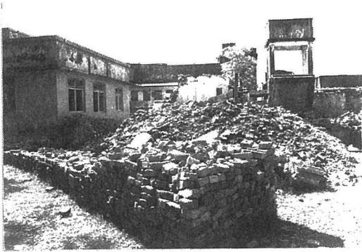
Photo. 3.28 Collapse of a brick masonry building: the nurses' headquarters, Dharan Hospital, Dharan Bazaar, Nepal
