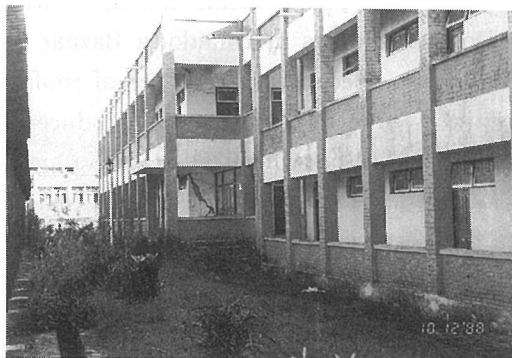
Photo. 3.34 Seriously and slightly damaged classroom buildings, the Engineering College Campus, Tribhuvan University, Dharan Bazaar, Nepal
