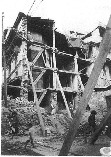
Photo. 3.10 Typical pattern of damage to a brick masonry building produced by the earthquake; example 1
