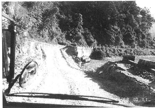
Photo. 3.71 Retaining wall failure
