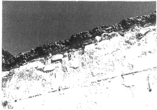
Photo. 3.2 Cross-sectional view of the floor slab system of the same damaged brick masonry house
