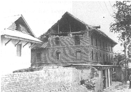
Photo. 3.38 Damage to the gable wall of a brick masonry building; example 3, Dhankuta Bazaar, Nepal
