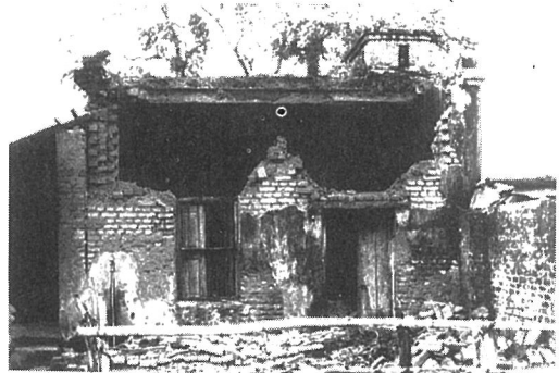
Photo. 3.21 Damage in the Darbhanga area, view 2 (courtesy of the Building Construction Department, Government of Bihar)
