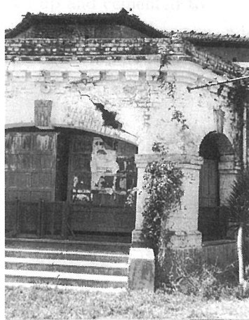
Photo. 3.16 The damaged Civil Sergeant's Residence, Darbhanga District, Darbhanga
