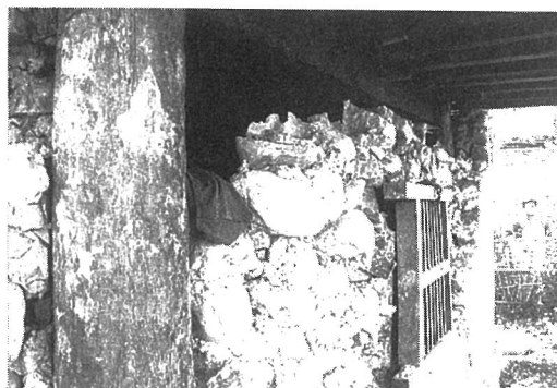
Photo. 3.9 A mud-stone, rural house at Gaighat, Nepal partly damaged during the earthquake
