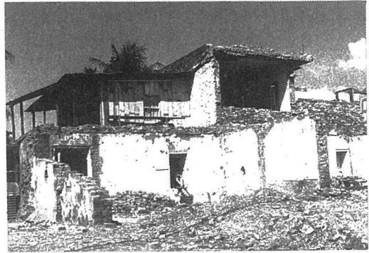
Photo. 3.29 A collapsed brick masonry house; example 1, Dharan Bazaar, Nepal
