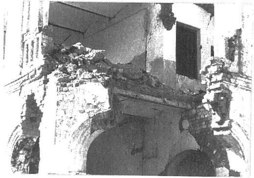
Photo. 3.18 Close-up of a cross-sectional view of the damaged Medical College Hospital, Darbhanga
