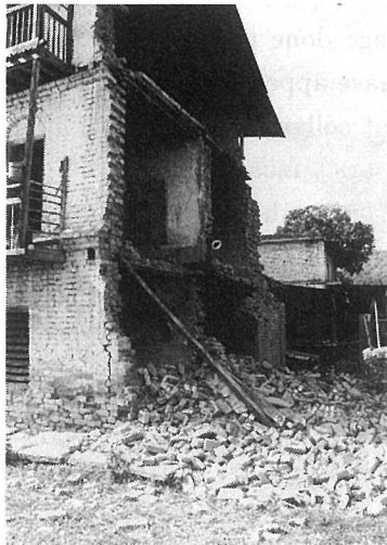
Photo. 3.11 Typical pattern of damage to a brick masonry building produced by the earthquake; example 2
