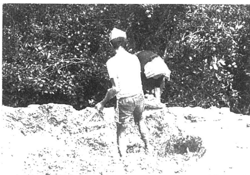
Photo. 3.7 Construction of a mud-stone house in Dharan Bazaar; mixing mud-mortar in the backyard
