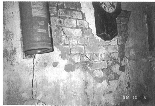
Photo. 3.15 Cracks on the brick masonry wall in the Darbhanga District Headquarters Office, Darbhanga
