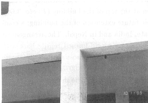
Photo. 3.59 Close-up of the top of the column of a third reinforced concrete private home, Dharan Bazaar, Nepal
