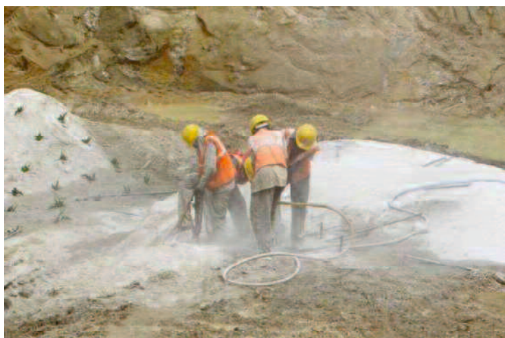
Photo 5-4 Poor environmental condition at the Indian construction site
