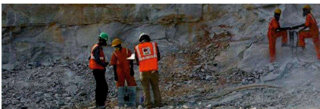
Photo 3-8 Daily site walk with the BMRC, the contractor, and the JICA team
