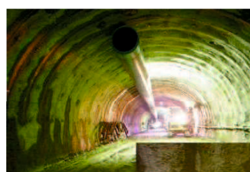
(a) Ventilation condition in tunnel
