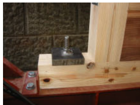
Photo2• Pedestal Junction Part
