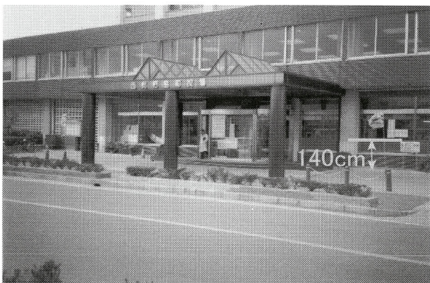
Photo 1. Flood mark on the glass of the door at the Nishibiwajima Town Office (Hanasaki-cho, Nishibiwajima Town).
