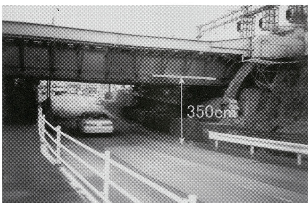
Photo 3. Flood mark under a bridge of the JR Tokaido Line (Yowa, Nishibiwajima Town).
