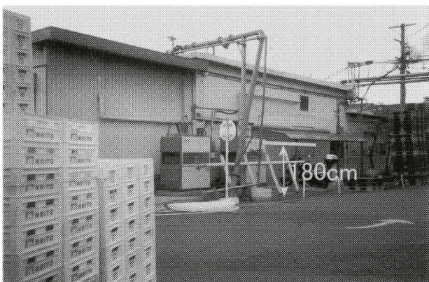
Photo 2. Flood mark on the wall of the Meito dairy factory located northwest of the JR Biwajima Station (Kaechi, Nishibiwajima Town).
