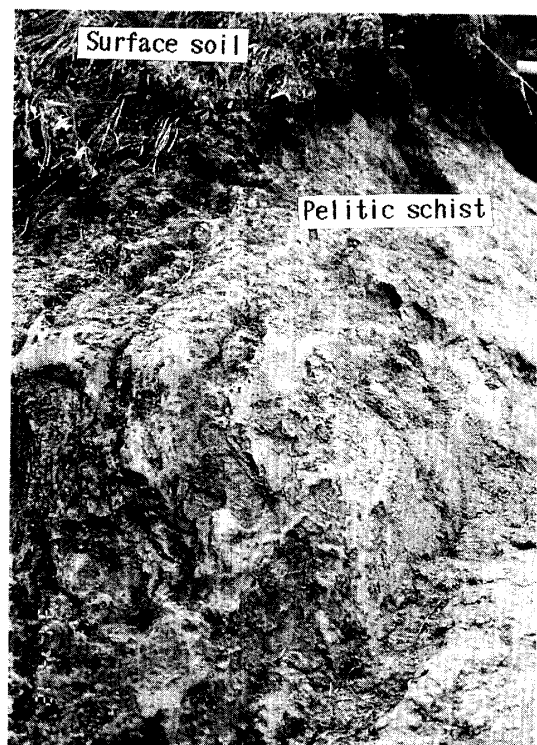
Photo.1 The state of failure of slope I
